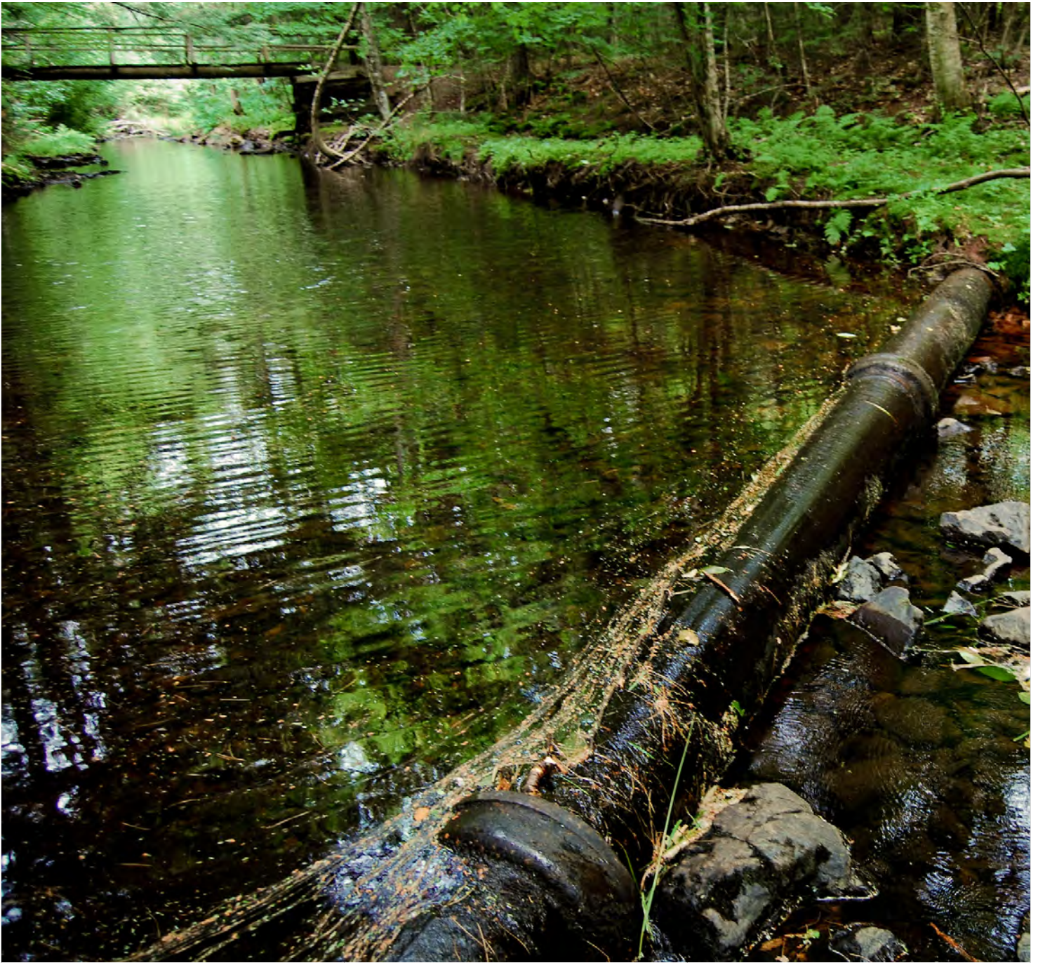
Pipe from reservoir impedes flow creating a pool.
